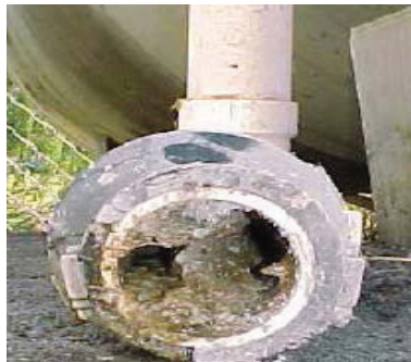
Figure 2. Blockages in Drain Pipe
