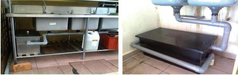
Figure 1. Example of grease trap installed under the sink
