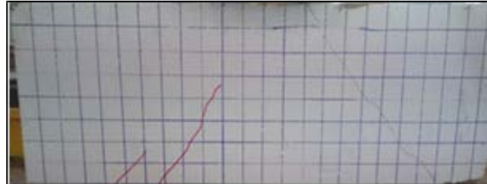
Figure 8. Crack pattern of reference beam, CB1
